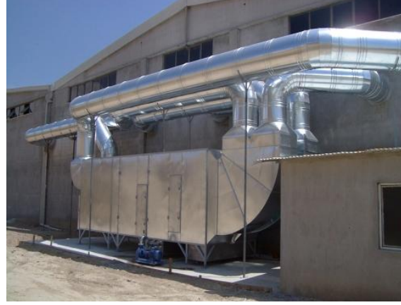
d) Klima santrali
